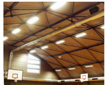
Gymnasium Winzerla - Germany, Aluform corrugated profile 55/177 perforated & smooth curved, rear side with acoustic fleece
